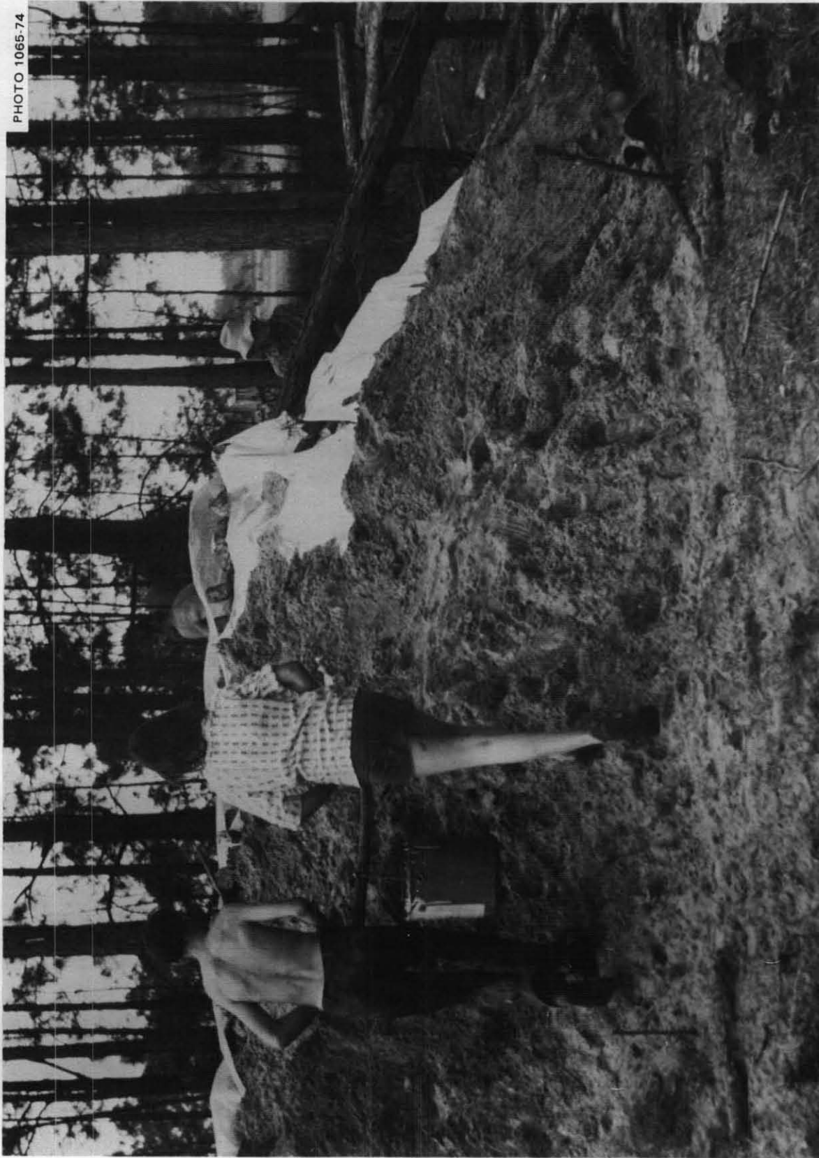
Fig. 5.36. Two teenagers carrying earth in a 5-gallon bucket, from one of the shallow barrow pits. These builders found that carrying earth in this manner enabled even children to move earth effectively, all the way to the top of the shelter.
